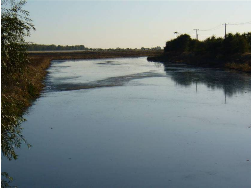
Raw sewage open inlet channel to lagoons with pumping station to WWTP1, and beginning of the lagoon system adjacent to WWTP1.
