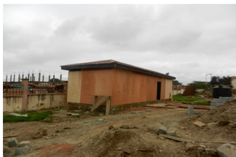
Construction of an environment-friendly biophil system in Amui Dzor communal sanitation block.
